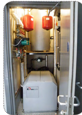
Heat pump and tanks located in internal storeroom.
