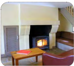
Pellet burner stove inside cottage
