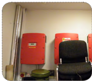
Wind turbine cabinets, located in internal storeroom.
